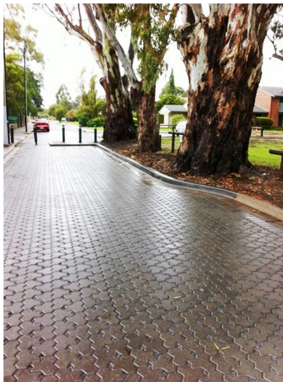
Figure 2. The absence of roots in road base material allowed its excavation without harm to nearby trees. Underdrains soak storm water from beneath the permeable pavement into the adjacent reserve as well as into the road subgrade; this has eliminated runoff from the paved surfaces.
