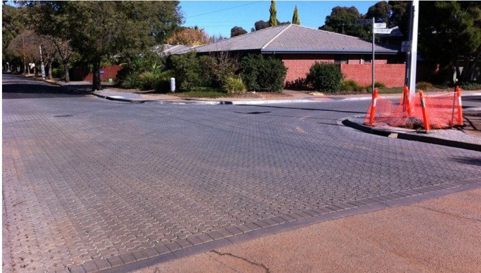
Figure 1. Permeable paving infiltrates stormwater into the road subgrade at the intersection of Kegworth and Wheaton Roads in Melrose Park, South Australia. As part of a broader treatment, this solution cost $1M less than the alternative option of upgrading the pit and pipe network.
